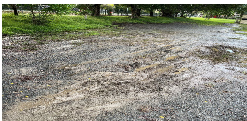
Figure 8 - Car Park 10 days after rain event
