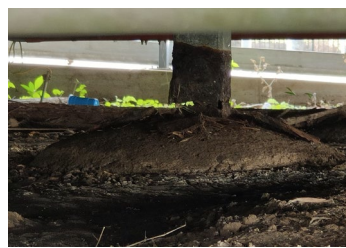
Figure 9 – Example Impact on building supports requiring building removal
