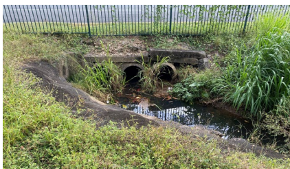
Figure 5 – School-side head wall degradation - potential to decrease flow restriction by covered pit. Access via grate or other
